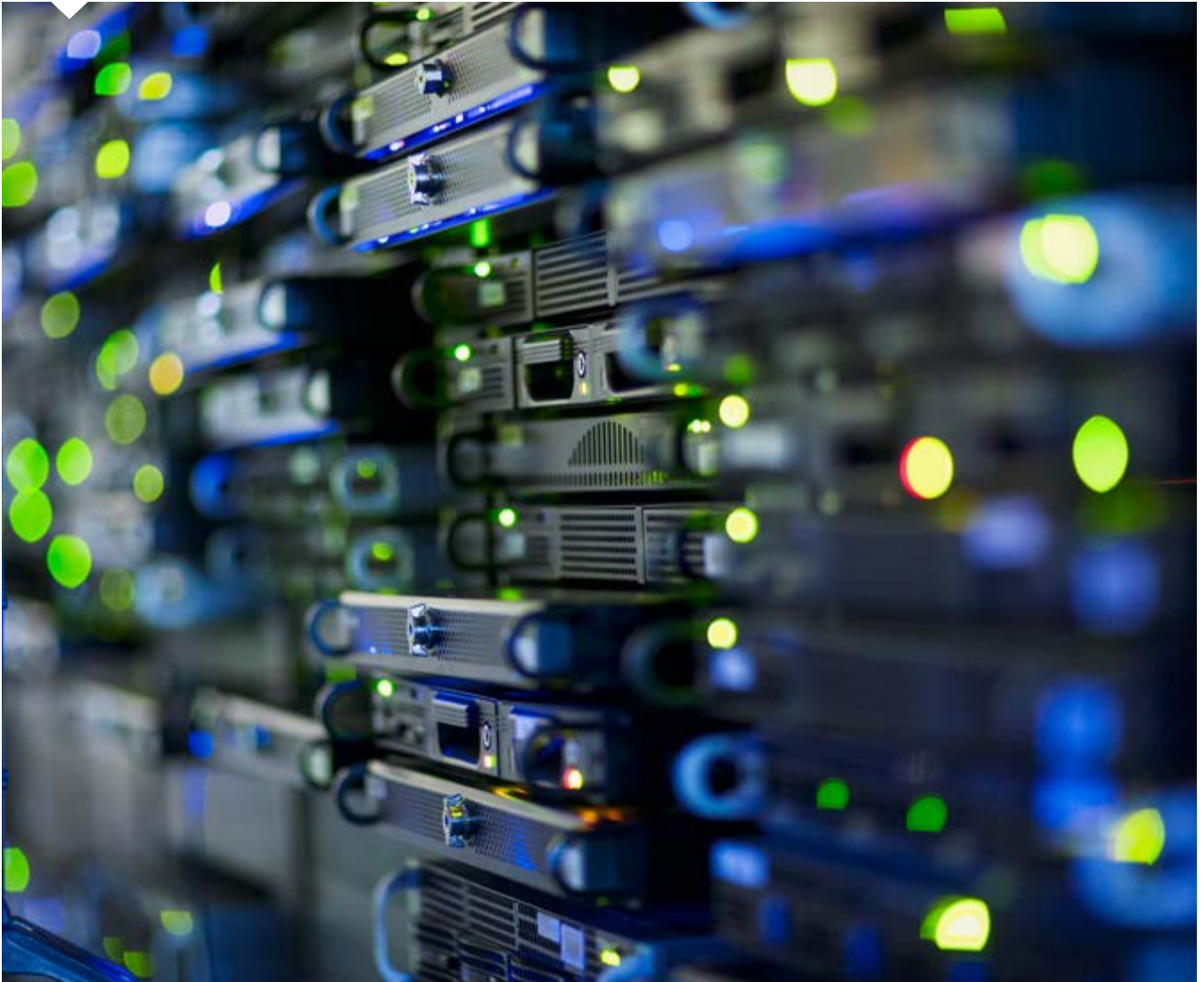
Server room rack panel
