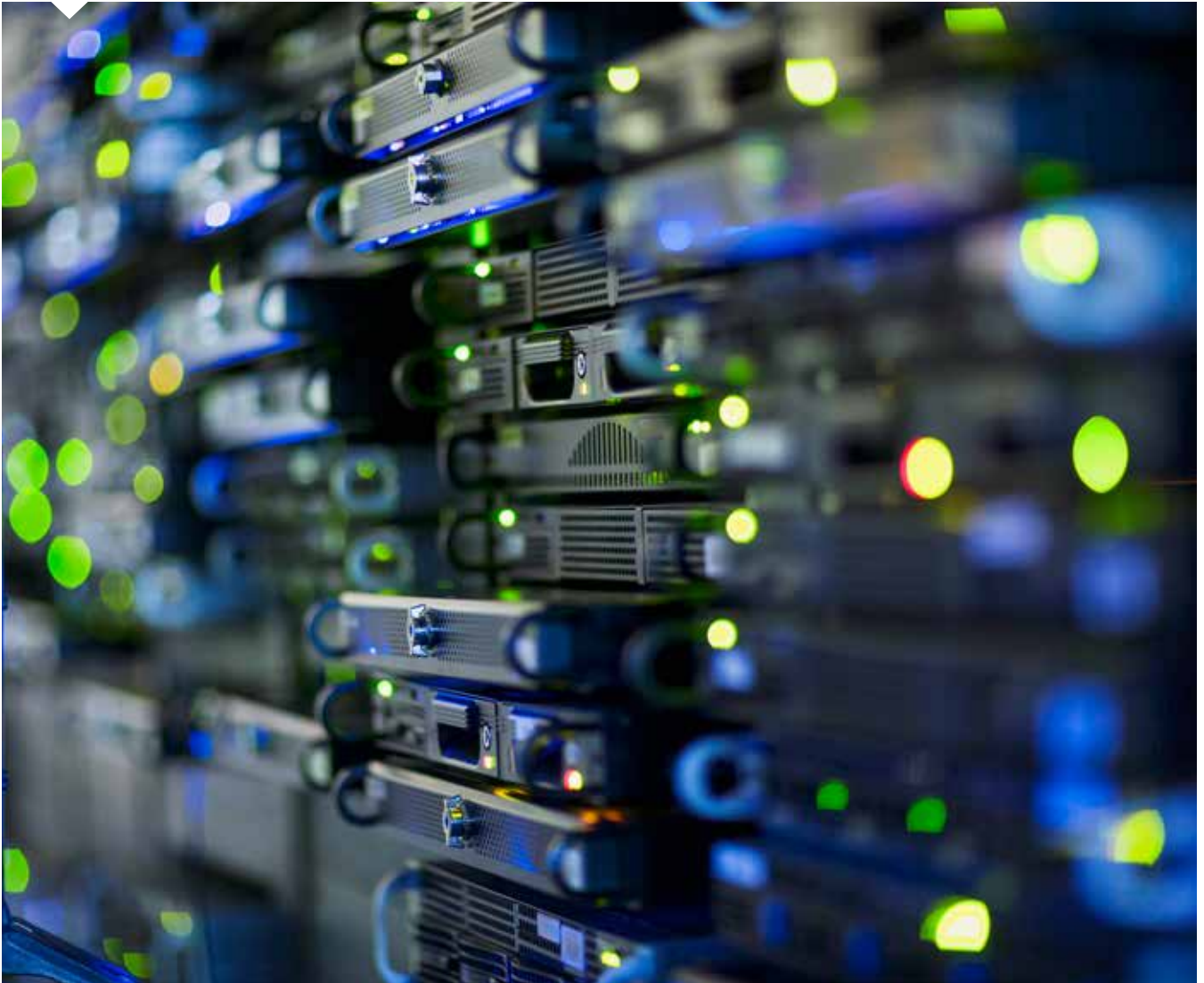
Server room rack panel
